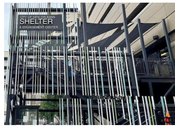
City of New Orleans Low Barrier Shelter 40,000SF Construction Interior build out to increase the current shelter's capacity by 200%.
